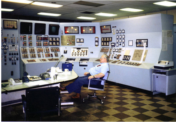
Minimum human intervention is required to control many large facilities such as this electrical generating station.
